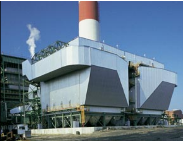
Precipitator with 16-inch wide plate spacing on a 320-megawatt coal-fired power boiler
