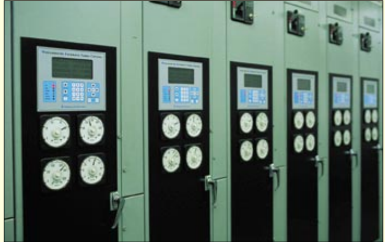
Automatic Power Control
