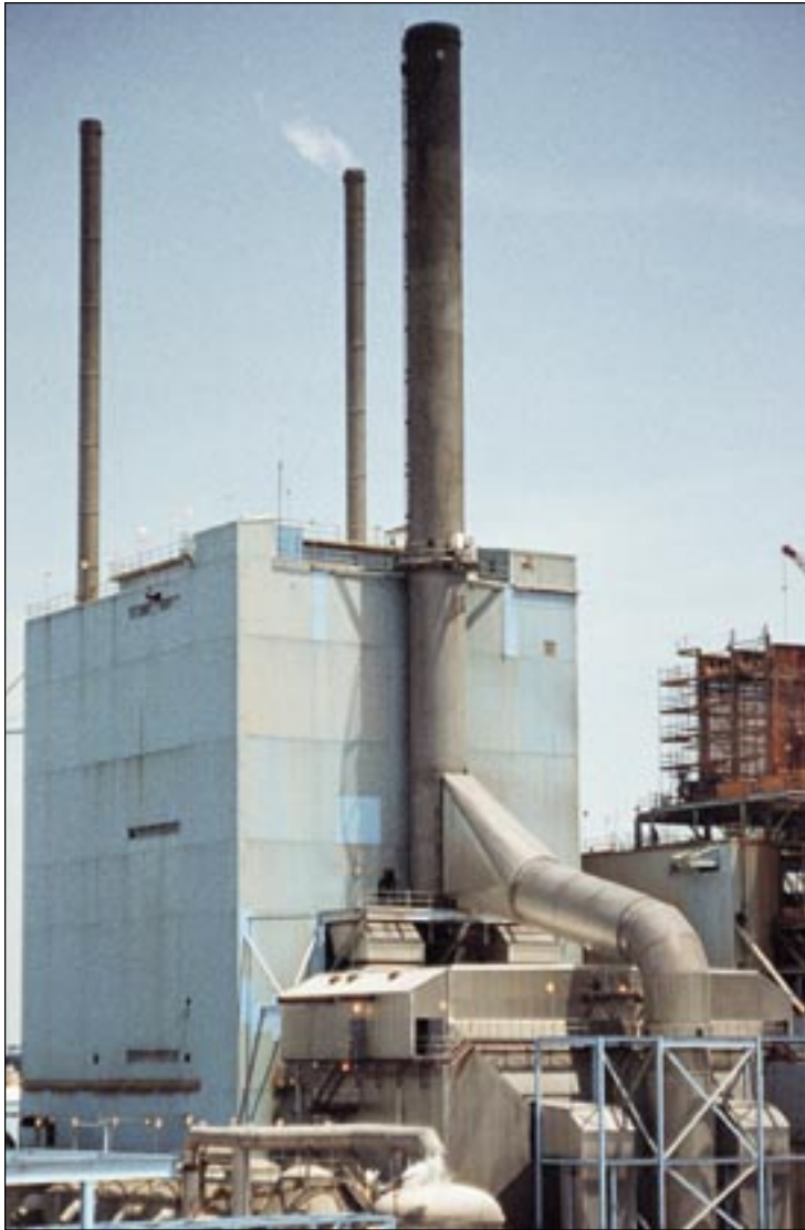
Pulp and paper recovery boiler
