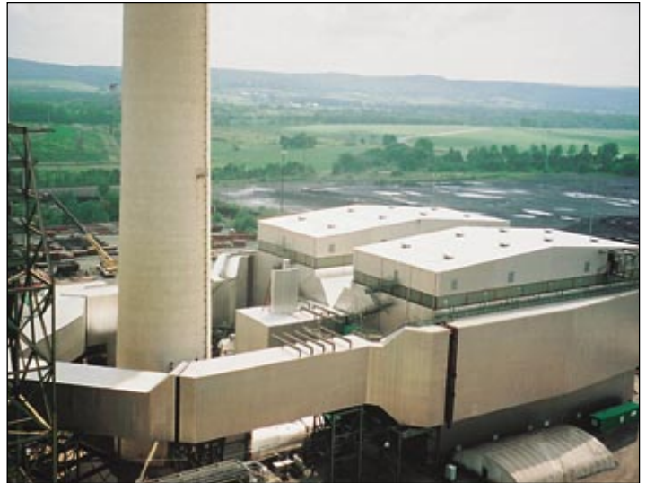
Two 745-megawatt coal-fired power boilers
