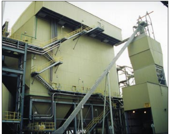
Pulp and paper power boiler
